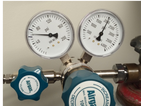
Nitrogen Gas Regulator (during operation)
